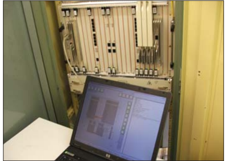
SDH Node Equipment at Otahuhu Substation
