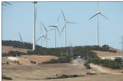
Mt Millar substation on the Eyre Peninsula in South Australia, surrounded by the Mt Millar Wind Farm
