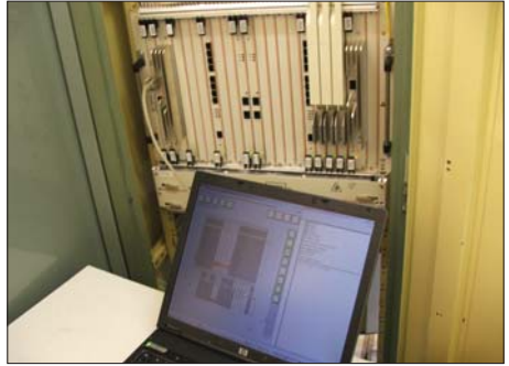
SDH Node Equipment at Otahuhu Substation
