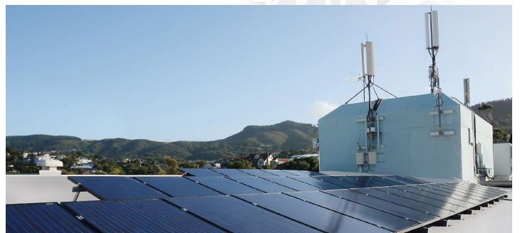
The PSC Solar array and PSC Audi e-tron
