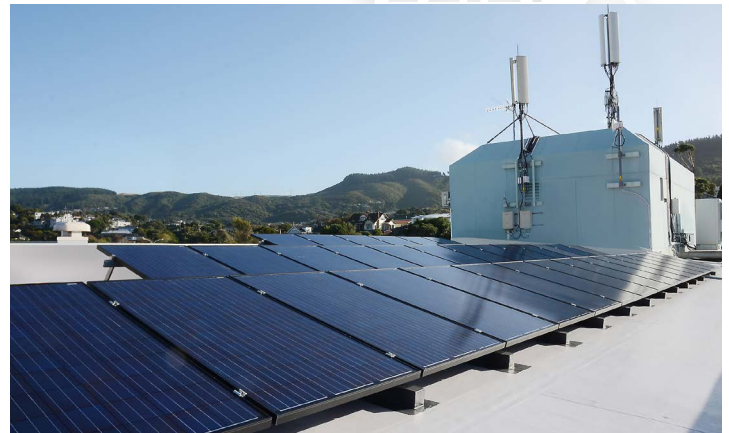
The PSC Solar array and PSC Audi e-tron
